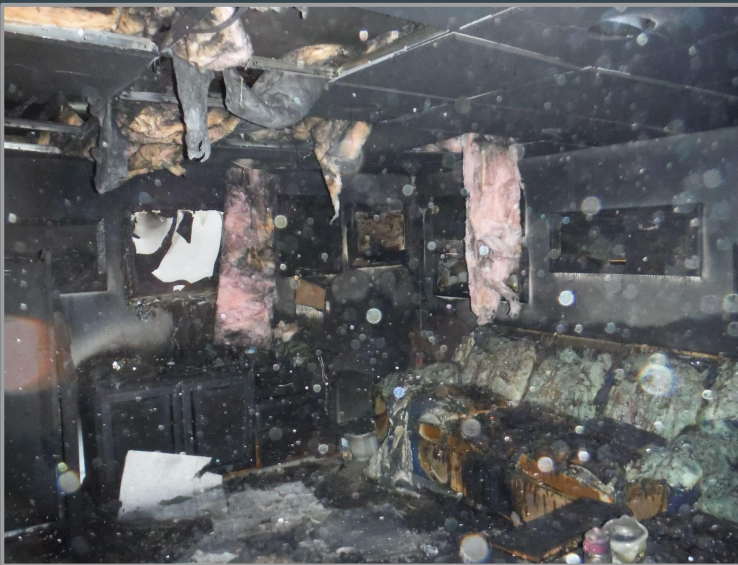
View of the finished basement looking at the couch that caught fire from the exploding battery (out of frame to the lower left)
