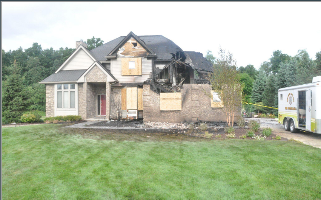
Post fire during the investigation
